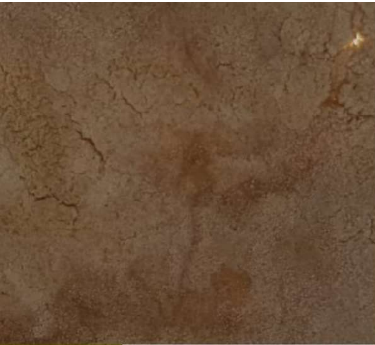
Cracking Wall Biometerial
